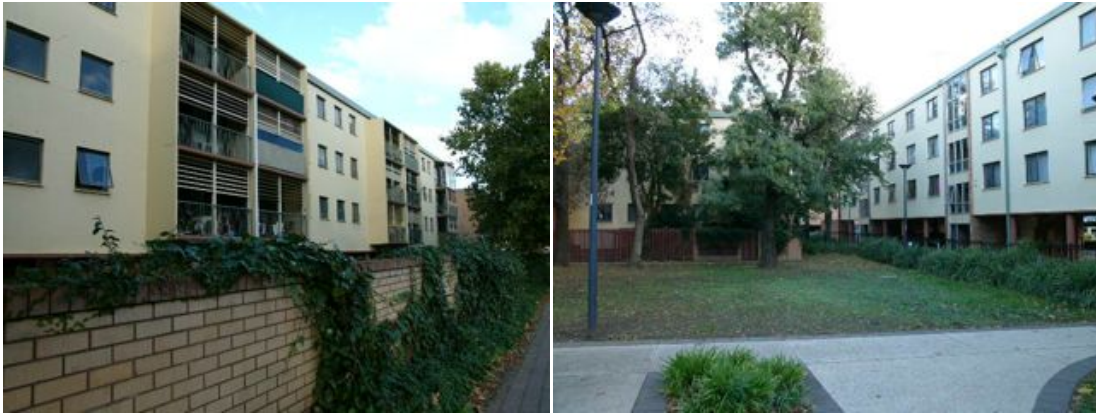
Illustrations 33 & 34: Allawah Court, flush-mounted square windows to south-west, north-west (partly obscured by trees) and north-east elevations, retro-fitted metal louvres to balconies. Photos by Milton Cameron, 2010.
